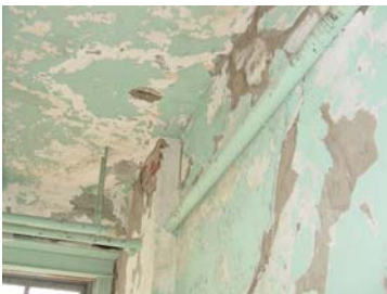
Photo: Peeling lead-based paint at a Philadelphia area residence in 2006.
